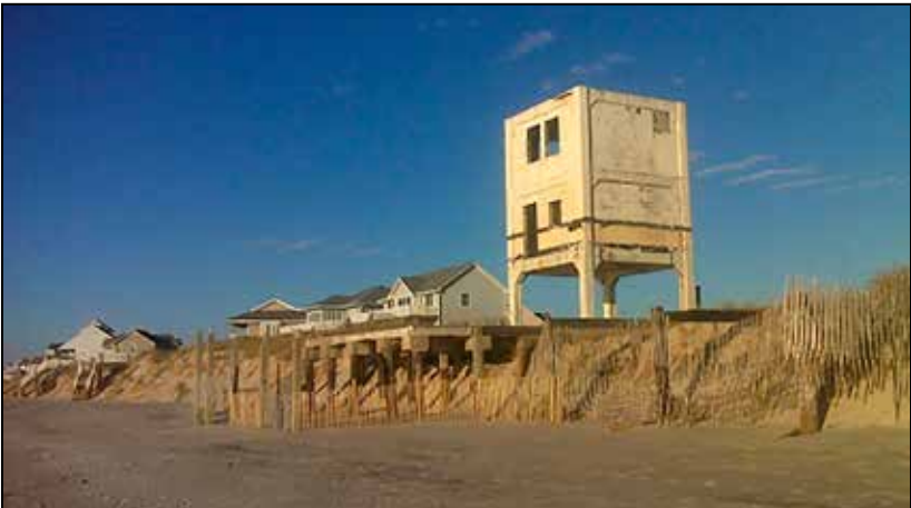
A 1946 rocket observation tower built for Operation Bumblebee Photo by PJ Wetzel, www.pjwetzel.com
